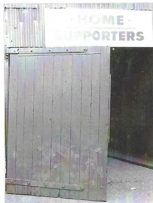
ENTRANCE GATES RIPPED OFF THEIR HINGES
